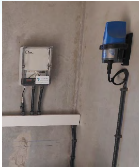
Figura 15 Elements de telecontrol i telelectura.
